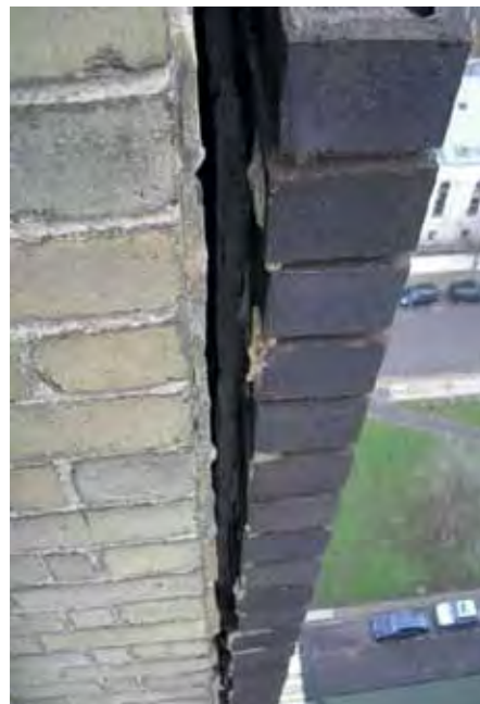
Figure 8: Brickwork in a state of disrepair and exposed concrete Source: Rockwool
