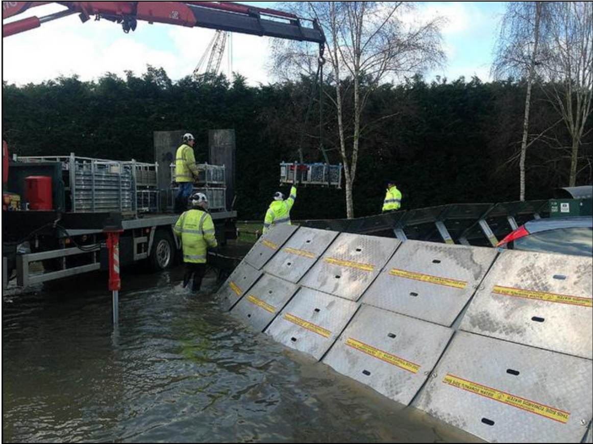
EA putting up temporary flood barriers in Caversham, November 2012. Photo courtesy of the Environment Agency
